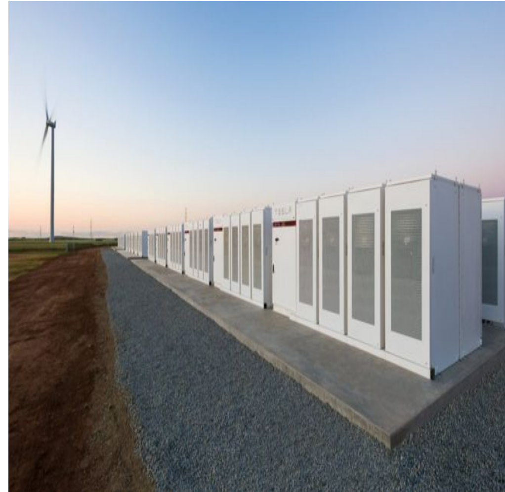
The world's largest lithium ion battery dispensing power into an electricity grid Jamestown, South Australia
