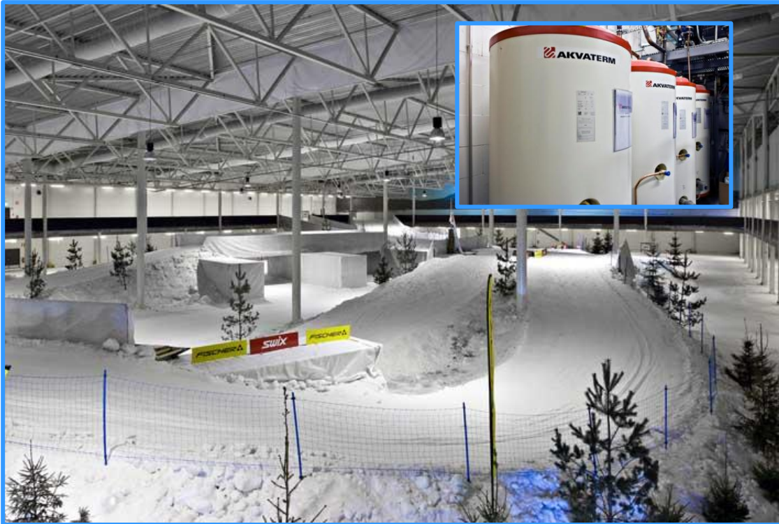
Winter sports arena cooling and heat recovery
